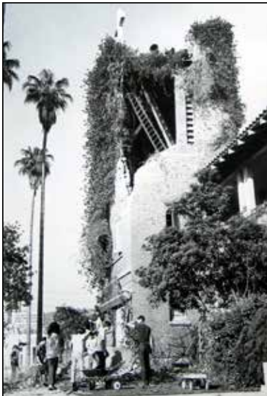
Damage to the Presbyterian Church Tower after the February 1971 earthquake. (ERVHS)
